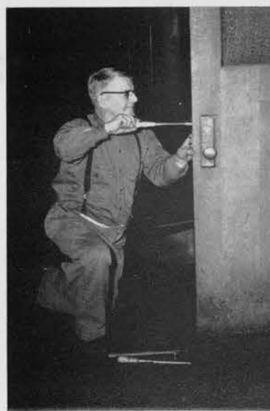
Below: Mr. John Foy does one last job of repairing a faulty lock before he retires.
